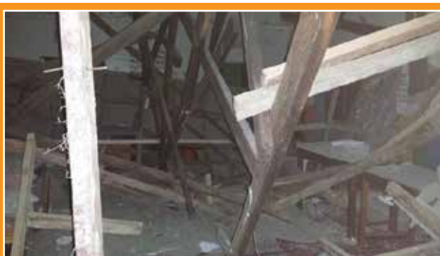
Classroom ceiling collapse in May 2016
